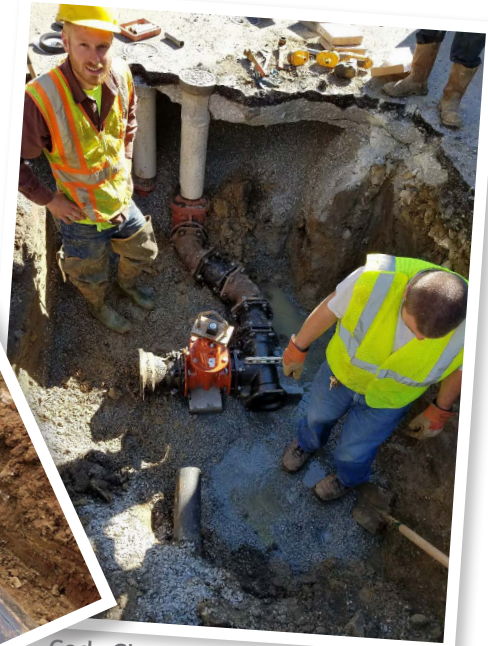
Cody Clark and Justin Miles install new water line on N. 4th and Flaget
